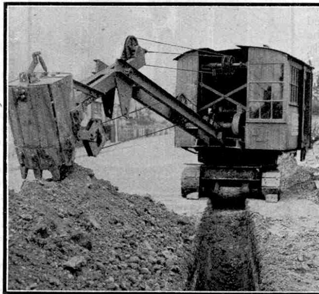
Cutting a trench through hard gravel with the aid of a "Universal" Trench Shovel.
