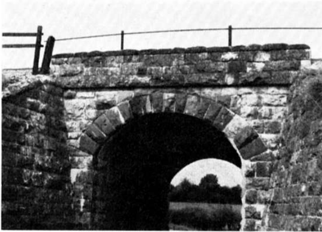
A 19th century stone arch bridge, carrying a railway line: this technique has remained unchanged after 2,000 years.
