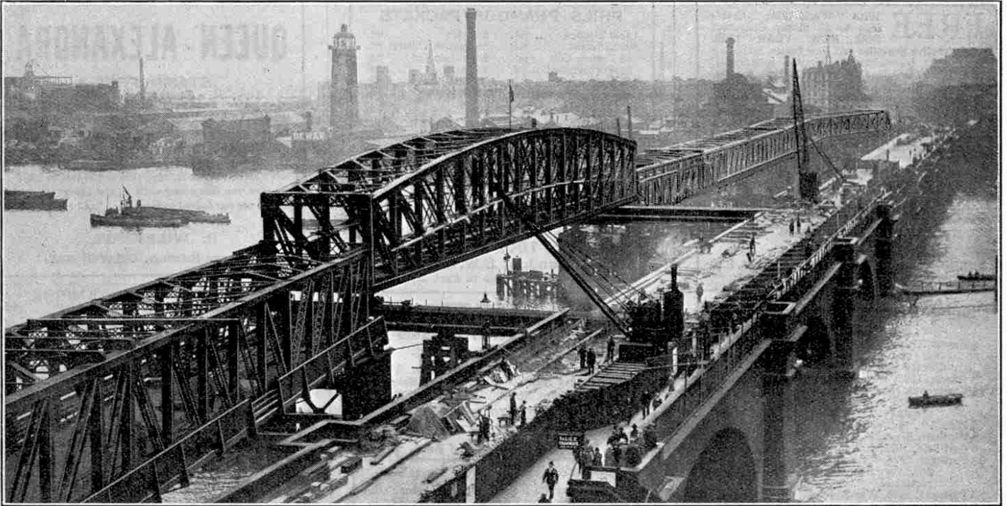
The Centre Span ready for lowering. It was raised and lowered by Hydraulic Jacks
