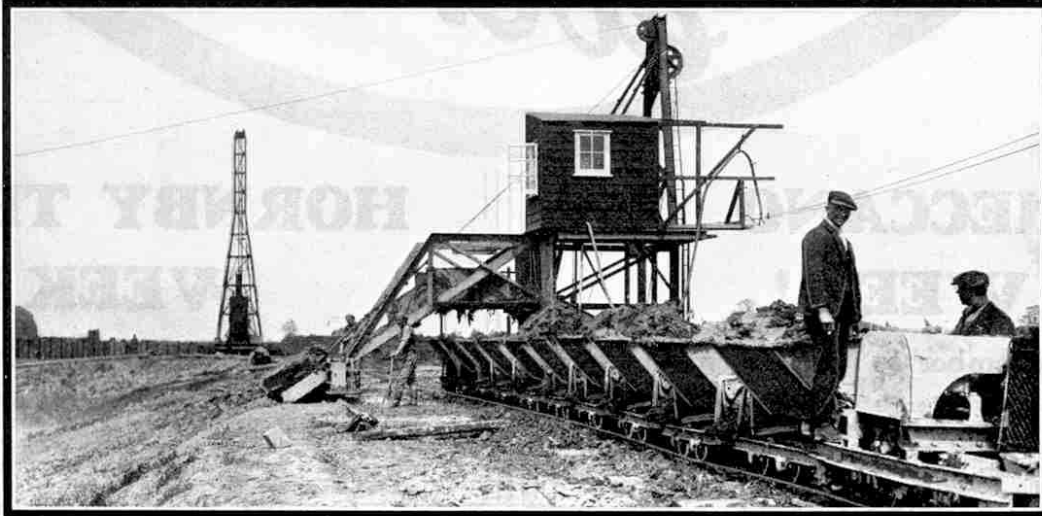
The head carriage of the Henderson Cable Drag-Scraper, with the bucket about to ascend the ramp. The tall structure in the background is a derrick. For this photograph we are indebted to the courtesy of John M. Henderson & Co. Ltd.
